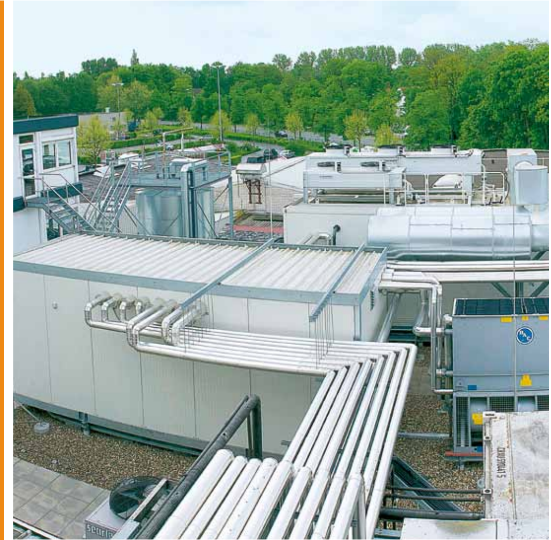
Top: The modular CHP plant is part of Mestemacher's power generation concept. It is connected to an absorption chiller and a steam generator with a downstream steam accumulator.
